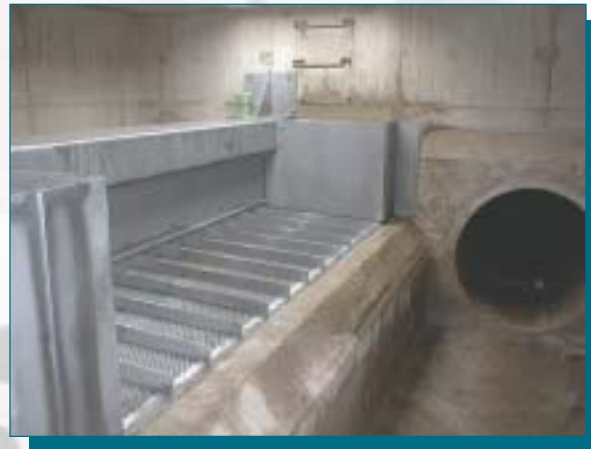
ACU-SCREEN in stormwater overflow basin.
